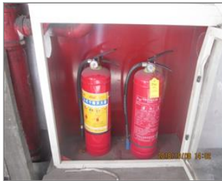
Photo of fire safety equipment Fire extinguishers.JPG
