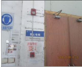
Photo of fire safety equipment Fire alarm.JPG
