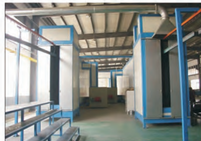
Dry off oven & curing oven
