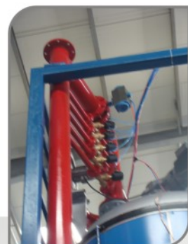
Multi-steam ventilation system
