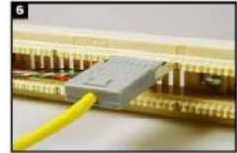
6 Insert patch plug into connecting block, and ensure them in tight connection.
