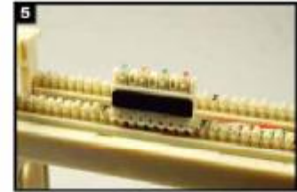
5 Checking the each wires following the color code on the connecting block's teeth.
